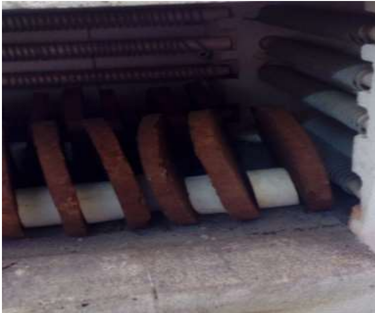
Figure 10: ceramic filters in a furnace
